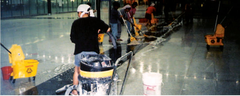
No Skidding® Anti-Slip Treatment was used on the new Hong Kong International Airport, the largest ever application of an anti-slip treatment. This terminal is designed to receive 85 million passengers annually. No Skidding® Anti-Slip Treatment was selected because of its effectiveness, ease of application, low maintenance and durability.
